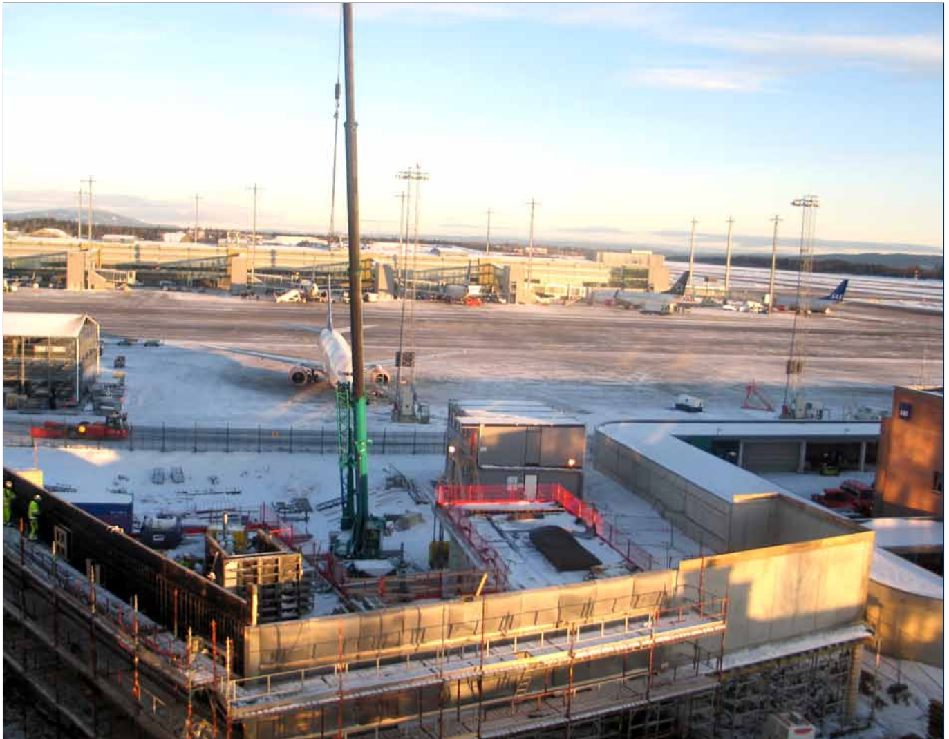
Construction of the new VIP house got underway in 2010 and will be completed during 2011.
